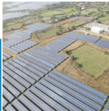
NTPC Nokh 306MWp, RJ
