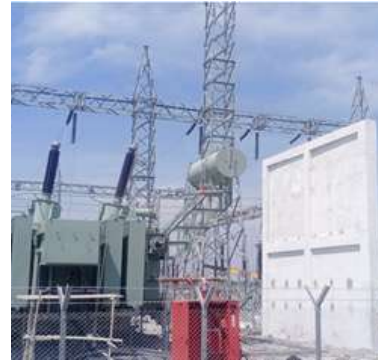
Statkraft 445MWp, RJ
